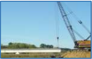
Mars Hill Bridge, Iowa First U.S. Highway Bridge using UHPC for precast UHPC girders
