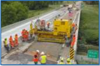
Floyd River Bridge, Iowa First machine laid U.S. UHPC Overlay for waterproofing and strengthening of bridge deck
